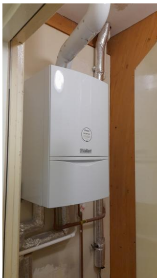
Existing 32kWth gas boiler for space heating
