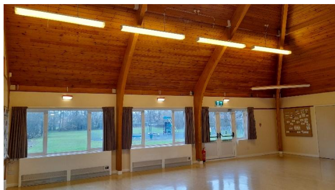
View of the main hall with existing linear fluorescent fittings
