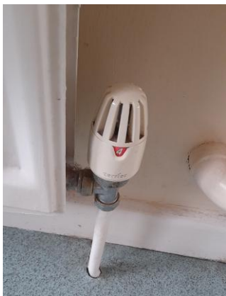
TRV on kitchen radiator
