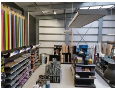
Example of electric IR heaters in high ceiling venue.
