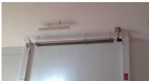
Existing gas radiant heater in the main hall at Acorn Centre.
