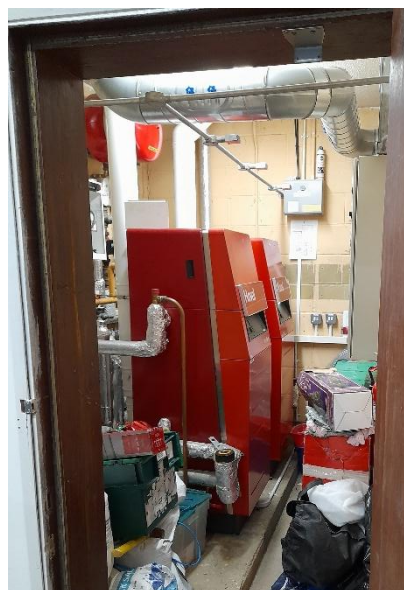
Existing 50kWth gas boilers for space heating and DHW.
