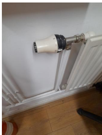
TRV at max setting on reception office radiator
