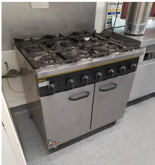
Existing hobs and oven natural gas unit in the main kitchen.
