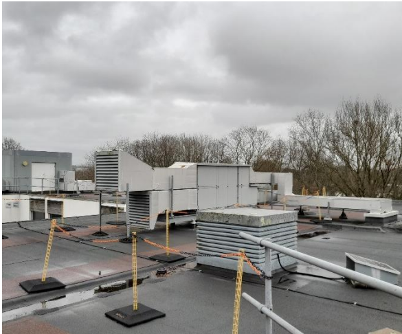
Example of roof top AHU.
