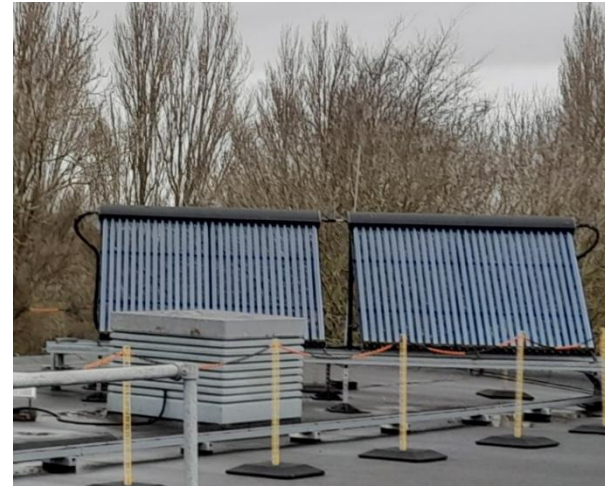
Hot water solar thermal collectors
