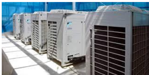
Example of ASHPs array.
