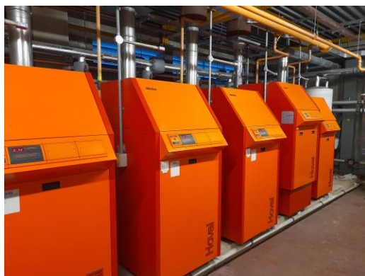
Existing gas boilers in blocks A&B plant room.
