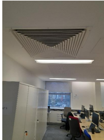
Example of T5 lights across open plan office areas
