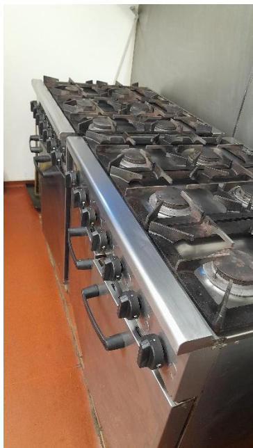
Existing gas hob and oven units in main kitchen
