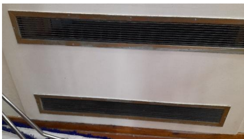
Existing wall concealed fan convectors in main hall.
