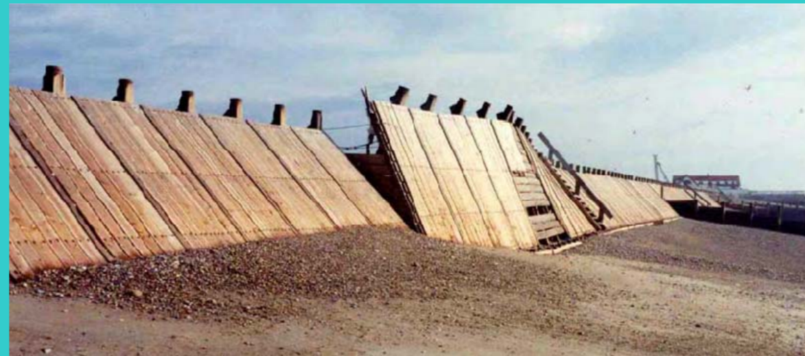
Significant structural failure, Feb '90
